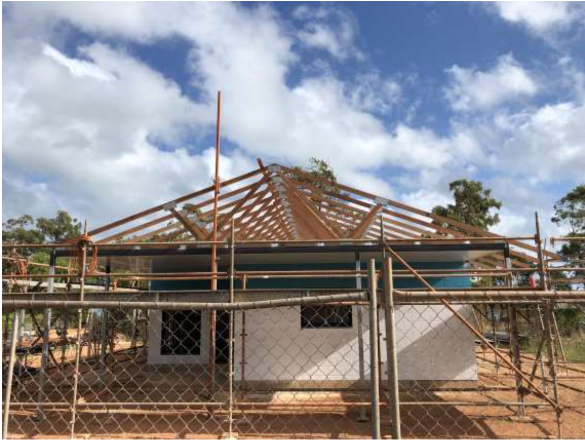
Gumatj hardwood truss being used for local housing, Nhulunbuy, East Arnhem, NT
